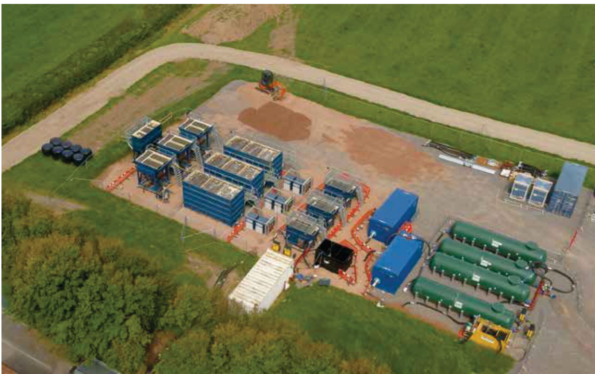
The Porlock Water Recycling Centre's existing membrane bioreactor facility was upgraded with a modular treatment solution provided by Siltbuster as part of the current capital program. The temporary works were delivered to site in February 2019 and remain in use in July 2020 as the MBR plant is being recommissioned. Photo credit: Siltbuster
