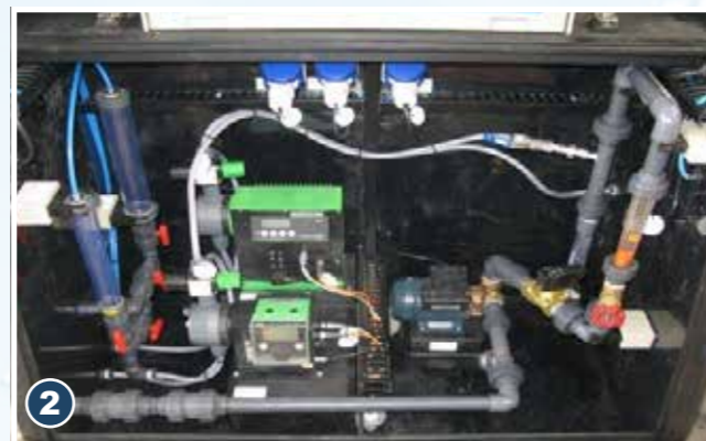
2 Proportional to the incoming flowrate, dosing pumps ensure the correct amount of chemicals are automatically introduced. Removing the risks associated with under/over manual dosing.
