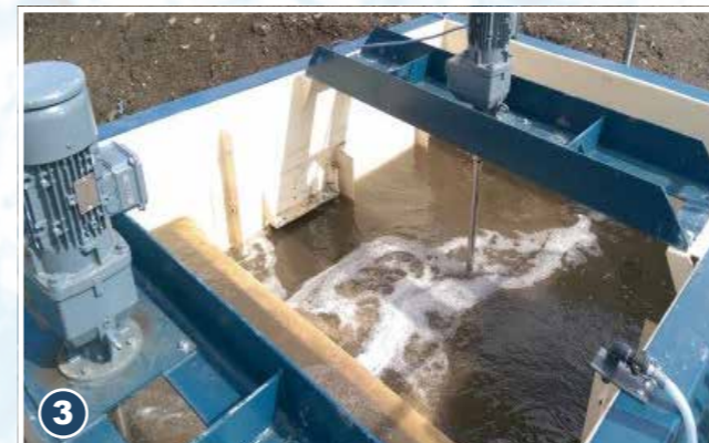
3 The chemicals are injected into a Mix Tank which provides contact time and mixing energy required to fully disperse and intermix the coagulant and flocculant.
