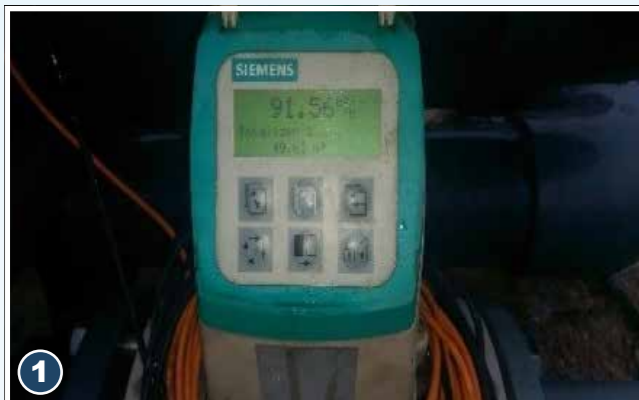
1 The incoming flowrate is measured in real time through the use of a digital magnetic flowmeter and relays the information to on-board chemical dosing equipment.
