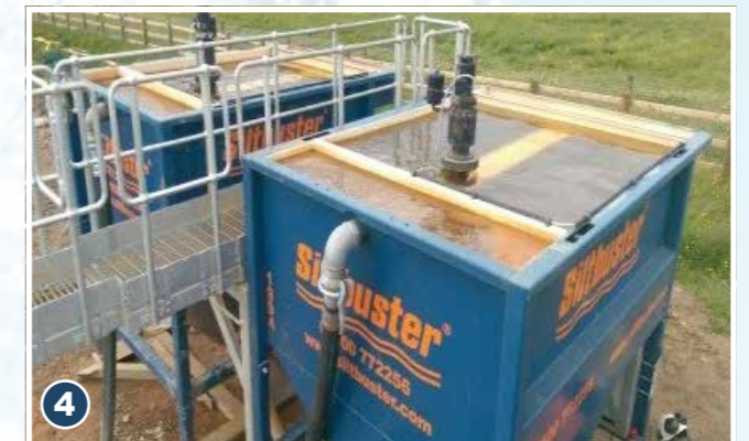
4 The chemically conditioned material then passes through an inclined lamella where the solids causing the waters to become dirty and discoloured are captured.
