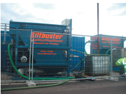
D20 DAF unit removing hydrocarbons on environmental remediation site
