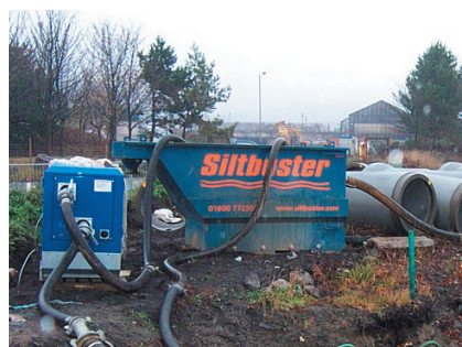
FB50 OWS unit treating ground water on construction site
