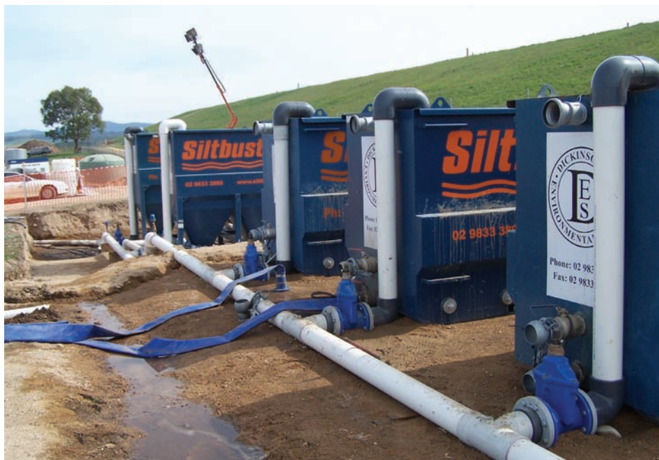
Siltbuster Clarifier units installed on site in Australia to help with water replenishment.
